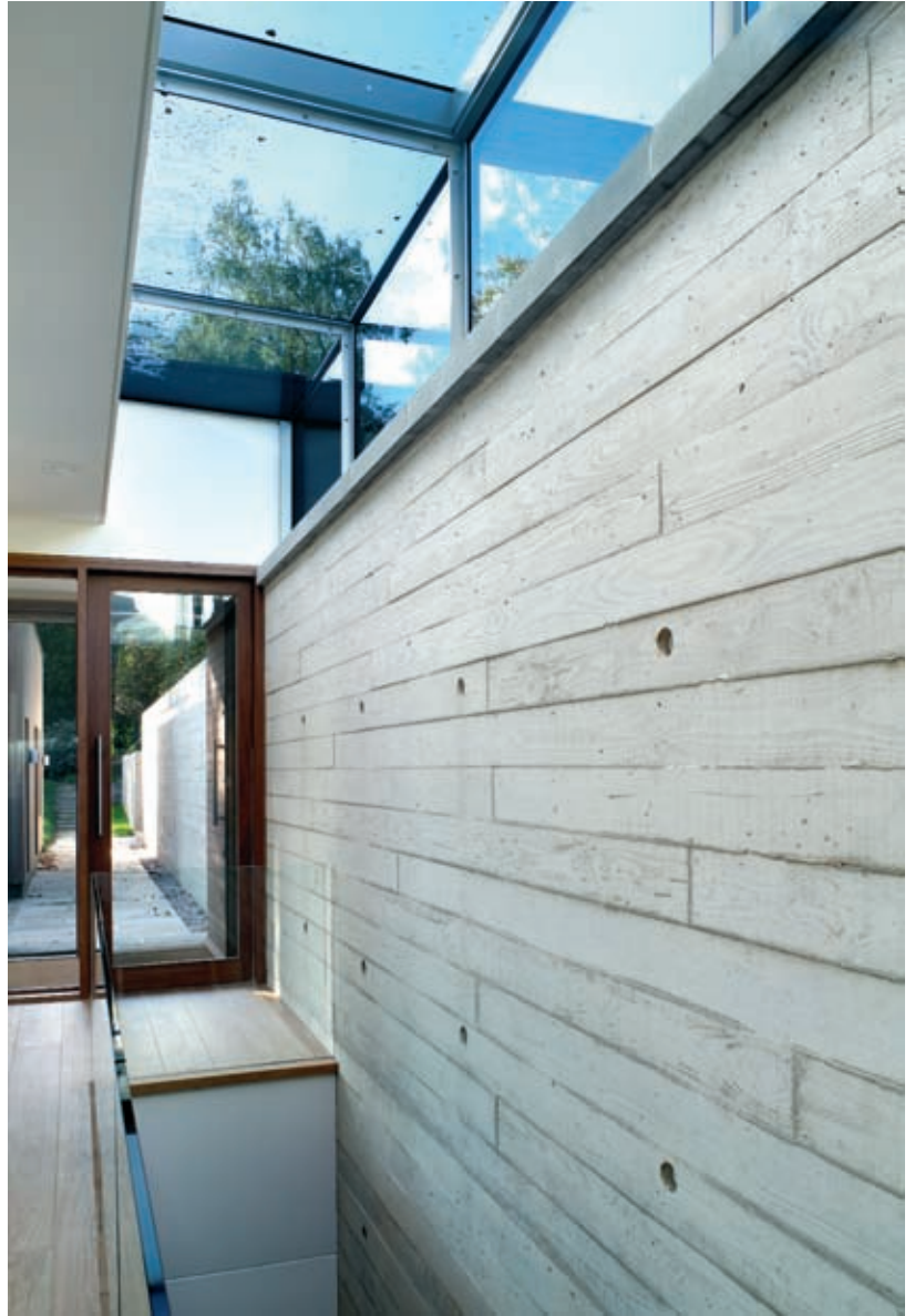
Above A full-height concrete wall acts as a thermal store.
